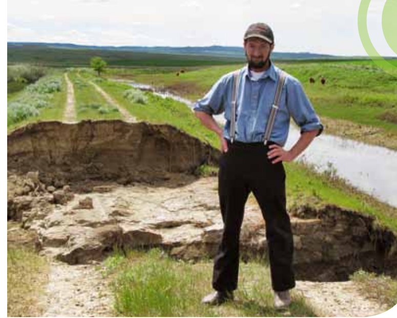
The irrigation works in the Cypress Hills region require ongoing maintenance. Repairs to this canal were required after washing out in June 2010.
